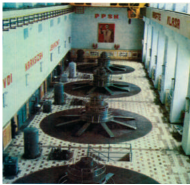
Doc. 89 Turbines' room at the Fierza Hydropower plant and Chemical plant
